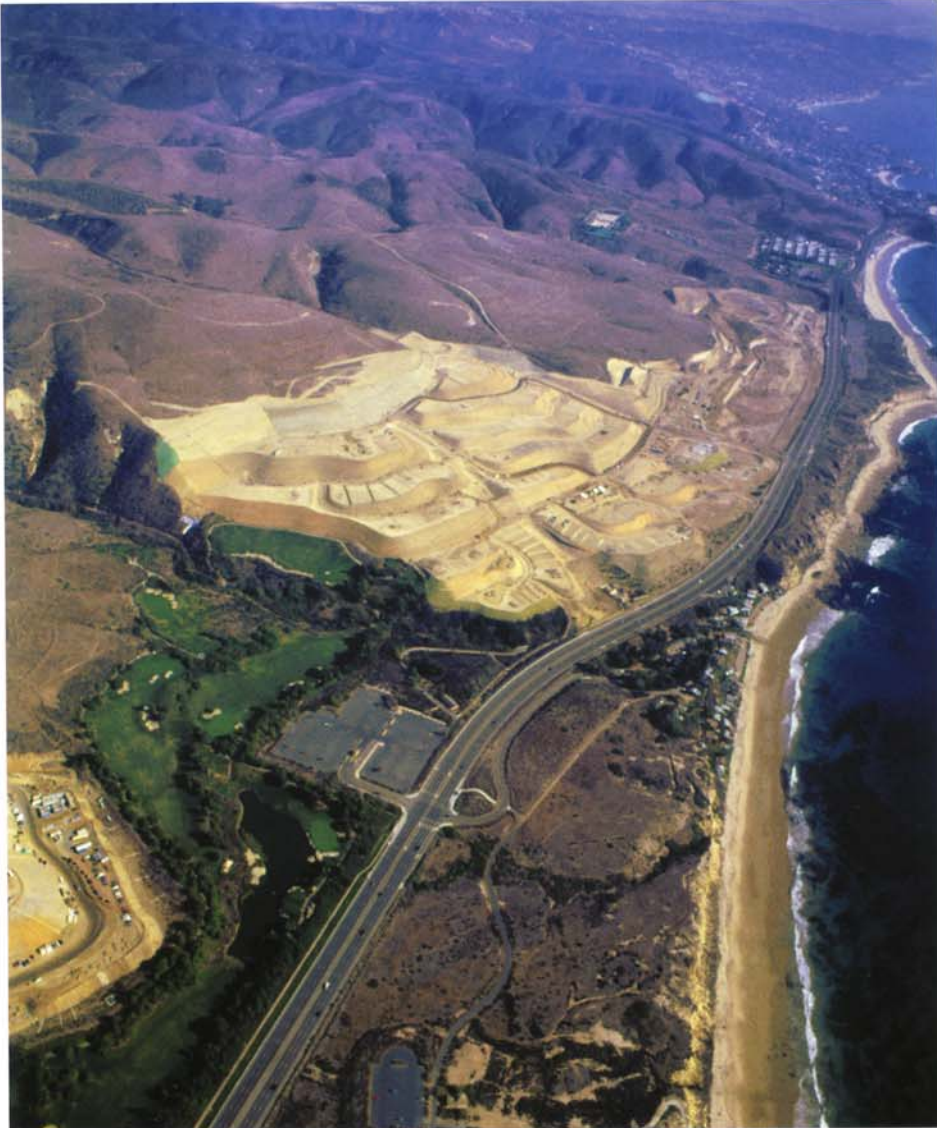
Great measures were taken to ensure some of the natural features on the Crystal Cove site were preserved like the Pelican Hill Golf Course and the natural slopes. The soil cement wall separating the golf course from the project is 55 feet tall, 8 feet wide and 1,000 feet long. Photo courtesy of Sukut Construction.
