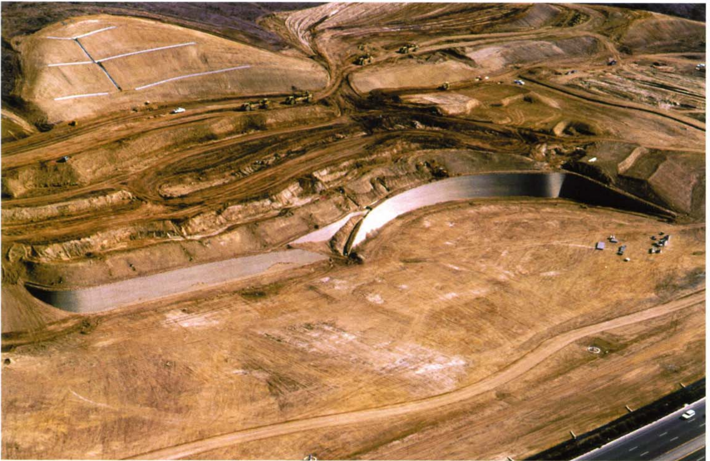
A new method of grading hillsides, developed by Soil Retention Systems, was used to install the 60,000 feet of retaining walls on the Crystal Cove project. Soil Retention Systems has mechanized the installation of modular block walls with a grapple machine designed specifically for the company. Photo courtesy of Sukut Construction.
