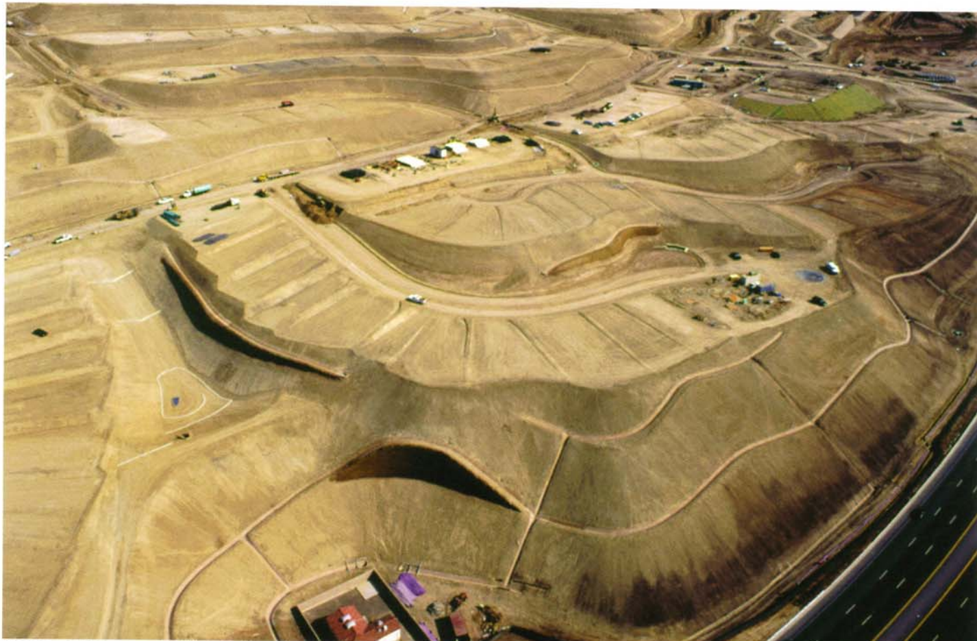
The Crystal Cove project involved moving 6 million cubic yards of dirt and the installation of a 1,000-foot long soil cement wall, 23,000 feet of reinforced concrete pipe, 60,000 feet of retaining walls, and 800,000 square yards of geogrids. The grading contract alone approached $20 million. Photo courtesy of Sukut Construction.
